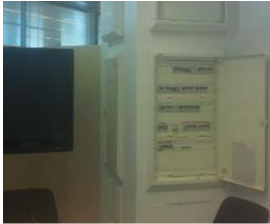
FIGURE 3: ELECTRICAL PANEL WITHIN THE 3RD FLOOR OFFICE, WITH CIRCUITS FEEDING FLOOR EQUIPMENT
